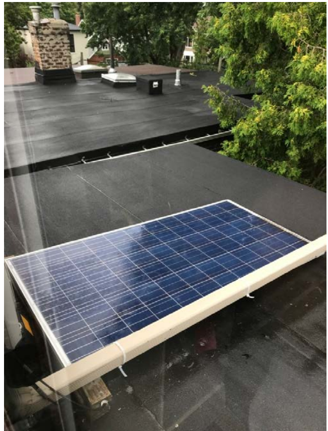
Figure 3: Rooftop Solar Panel 280W
